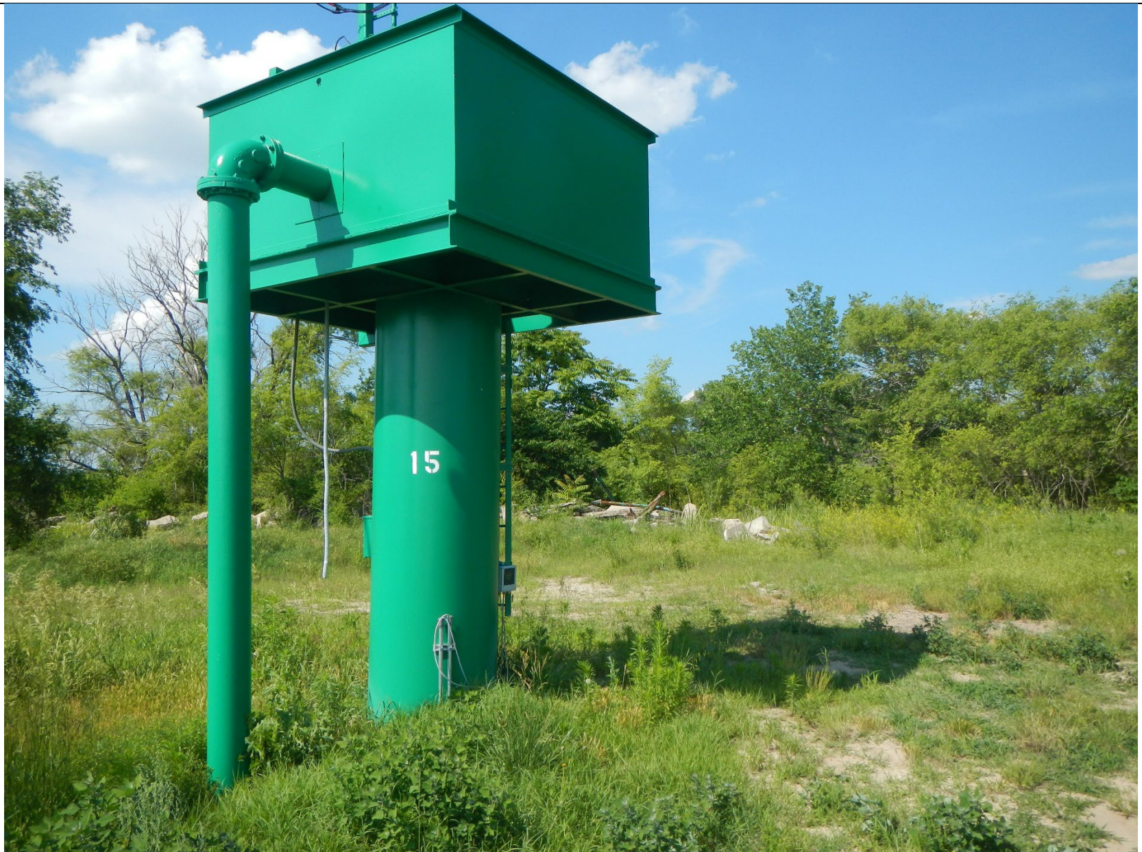
Overview of well #15, the Republican River is behind the trees.
