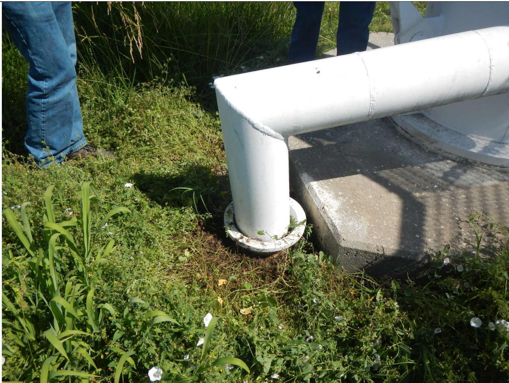
Spruce Street water tower overflow pipe. The pipe does not have a screen on it, and the air gap into the receiving pipe is inadequate.
