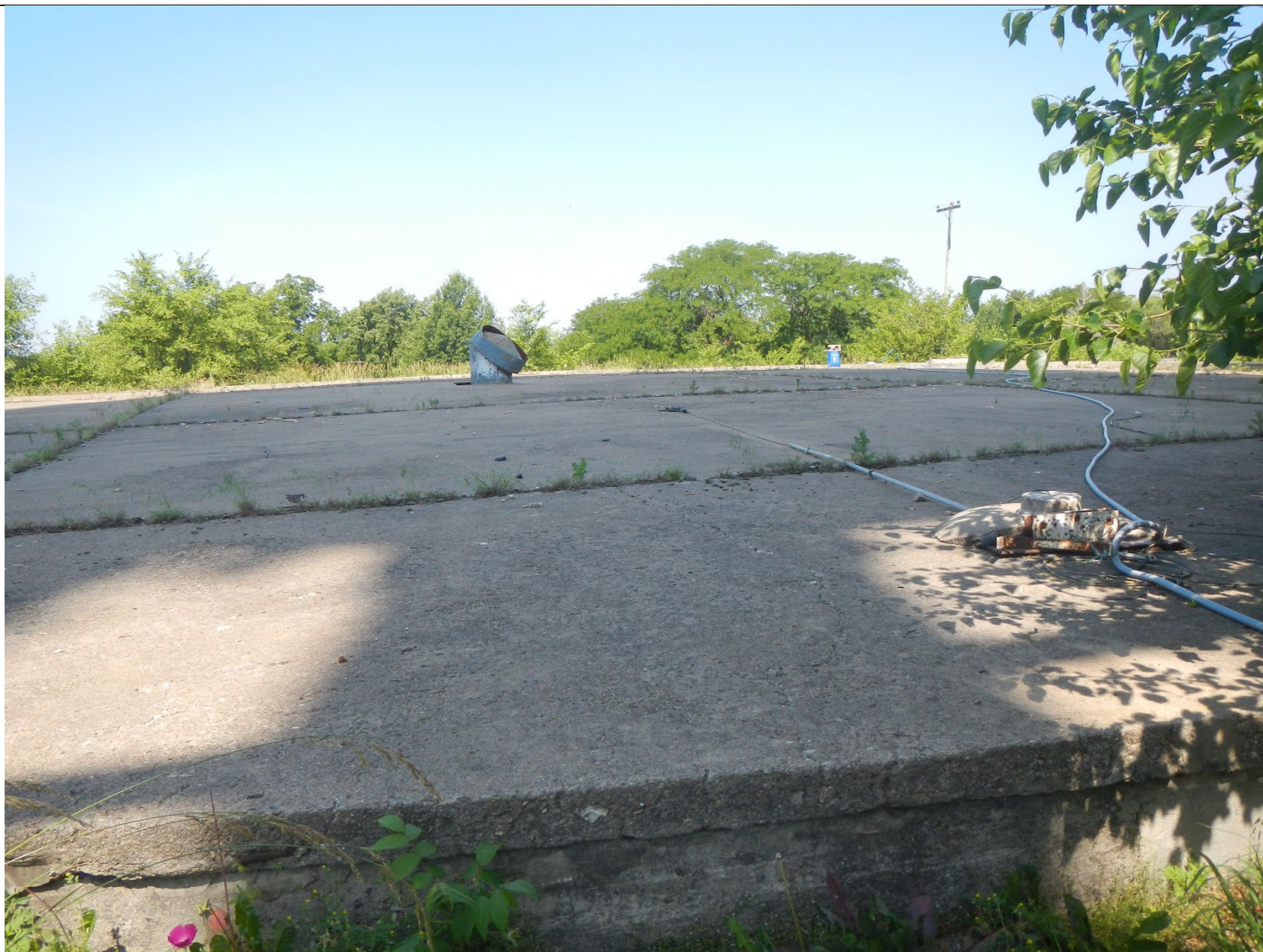
Overview shot of the top of the south ground storage tank. Broken vent lid in the center. Old level gauge and mounting bracket can be seen in the foreground of the photo. Raised access hatch from photo 23 can be seen in the background to the right.
