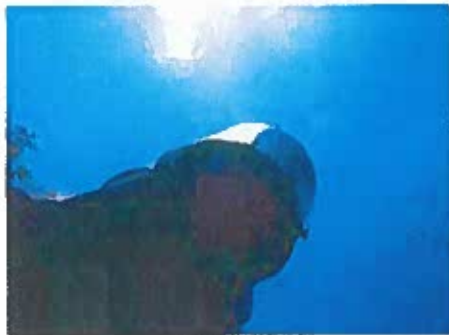
Well 015, air relief valve not screened
