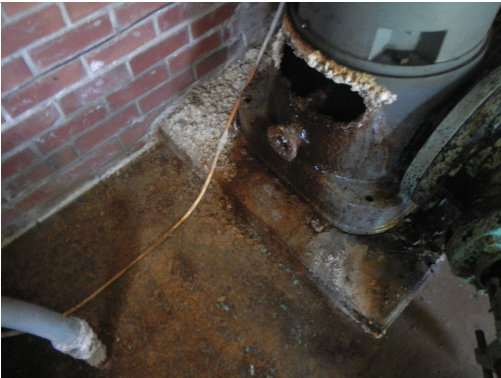
Excessive leaking from packing on booster station pump.
