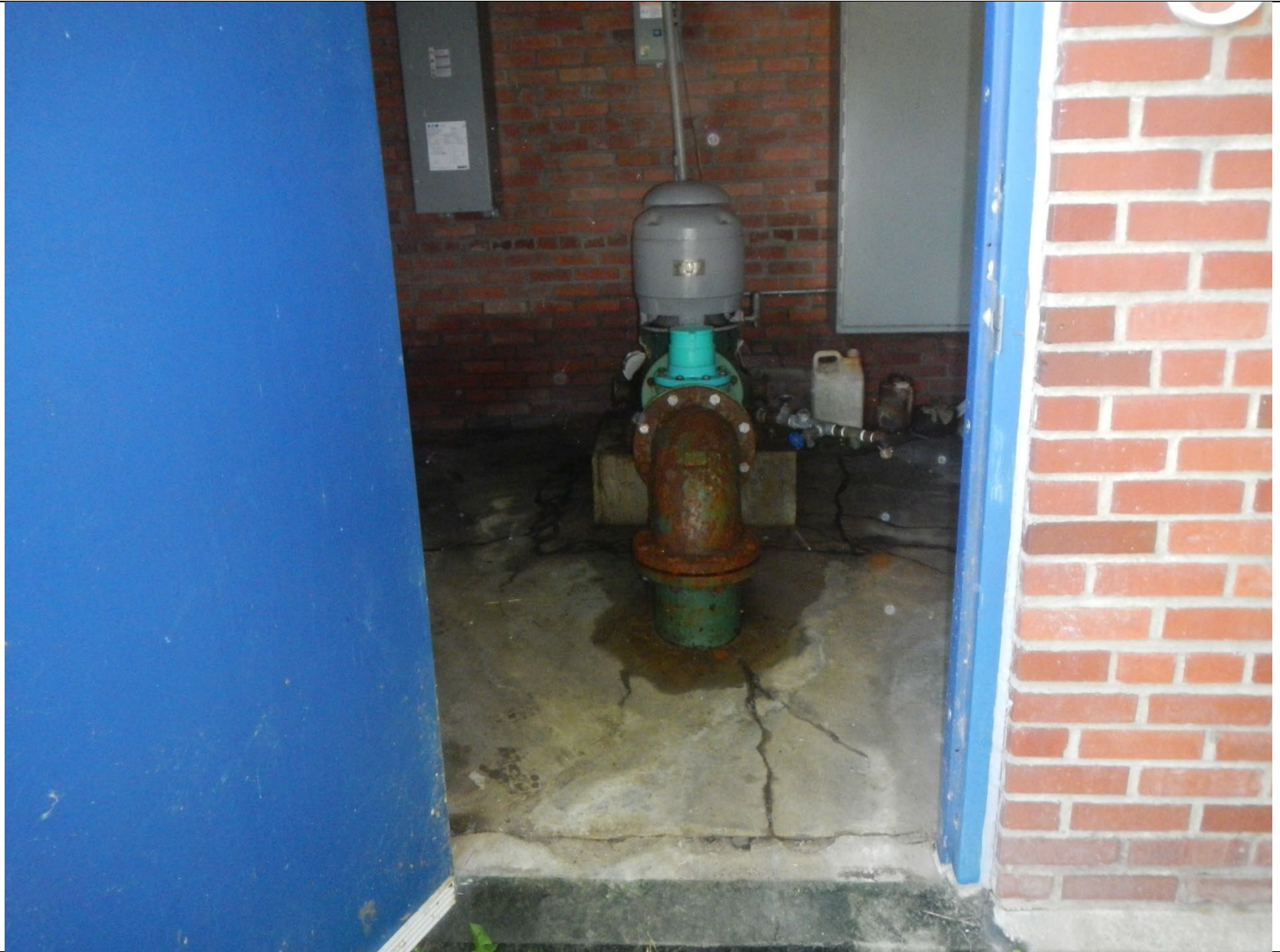
Well house and piping
