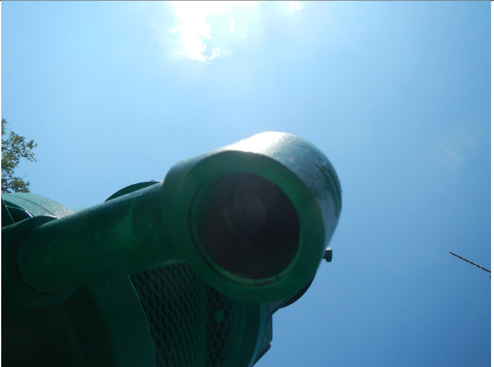
Unscreened well vent on well #17
