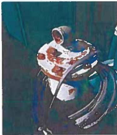
Well 015, air relief valve not screened
