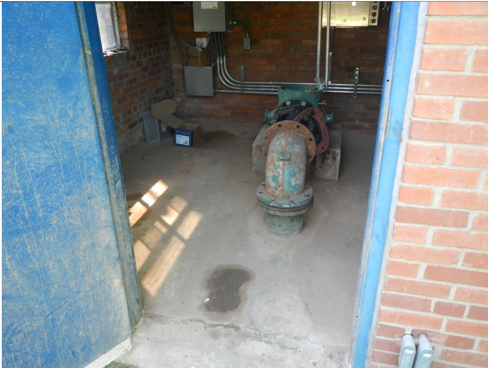
Well house and piping
