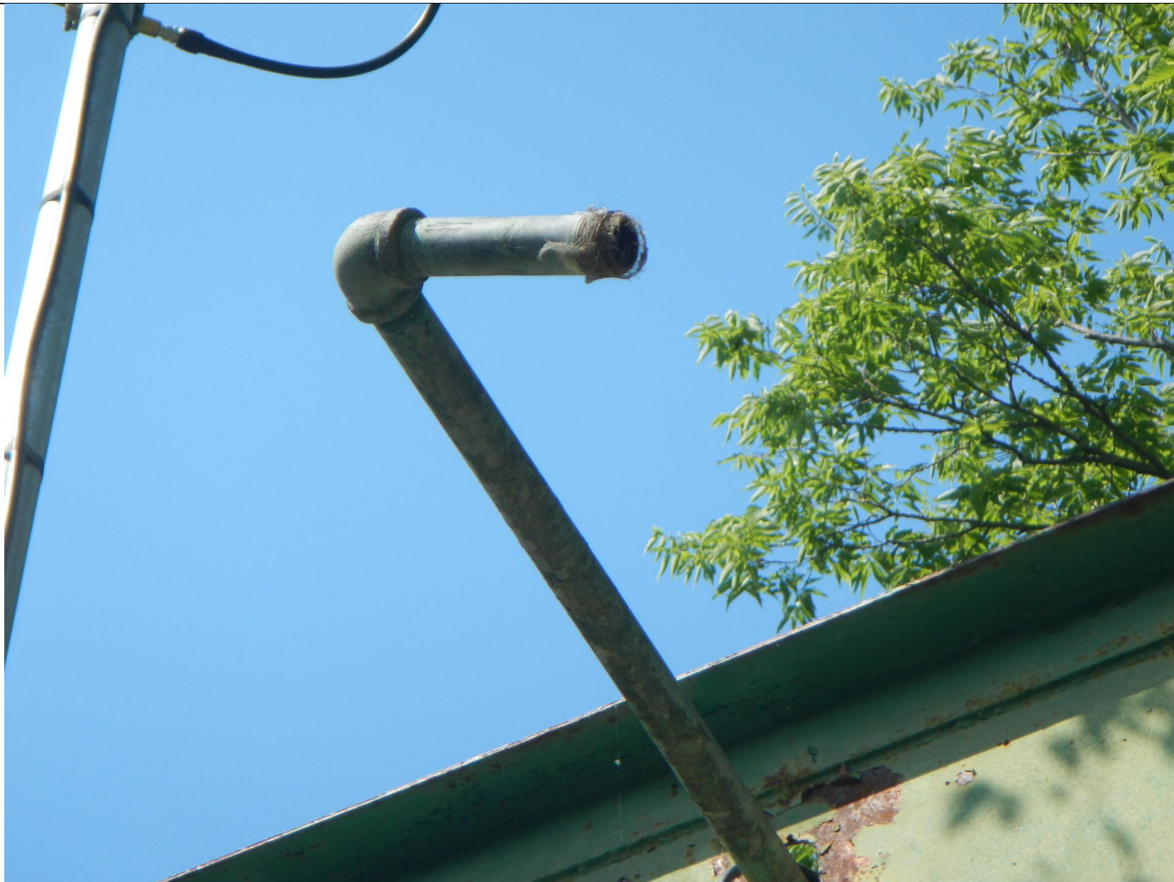
Air relief valve screen broken on well #11
