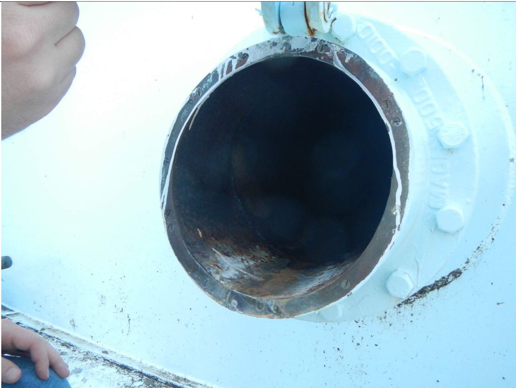
Overflow pipe on ground storage tank from photo 3. Pipe was not screened.
