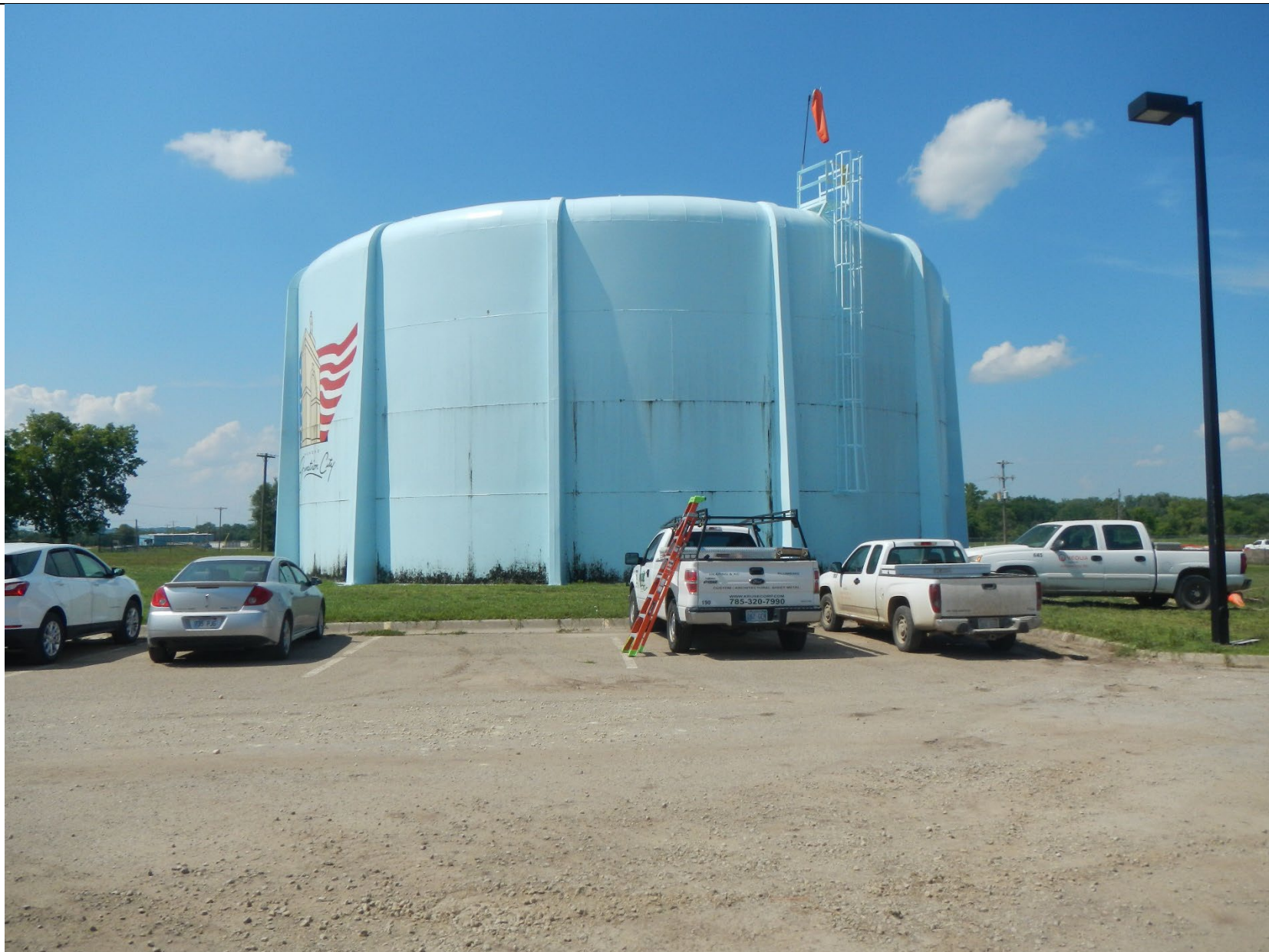
Finished water ground storage tank at water plant. Black material around base of tank is mildew.
