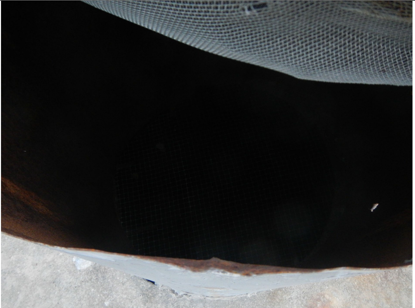
Gap in screen from photo 20 on the south ground storage tank vent.
