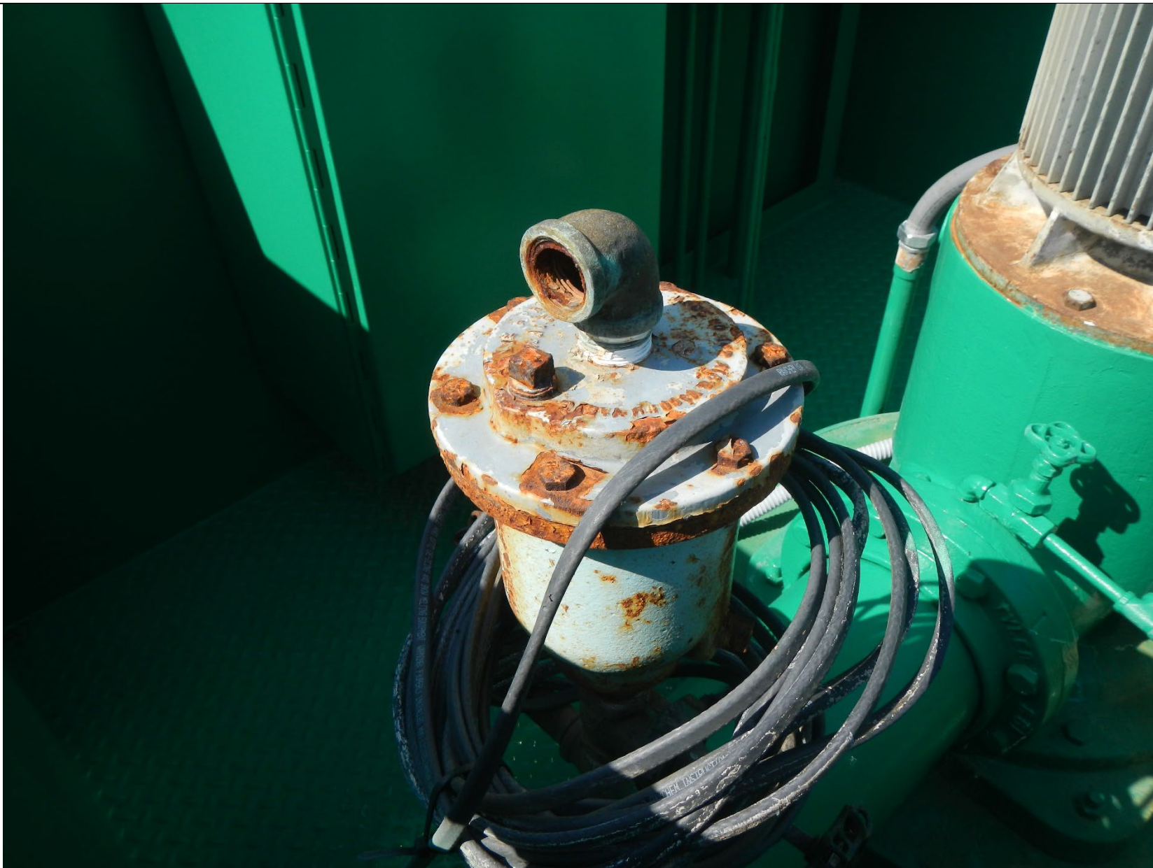
Well #15, air relief valve not screened.
