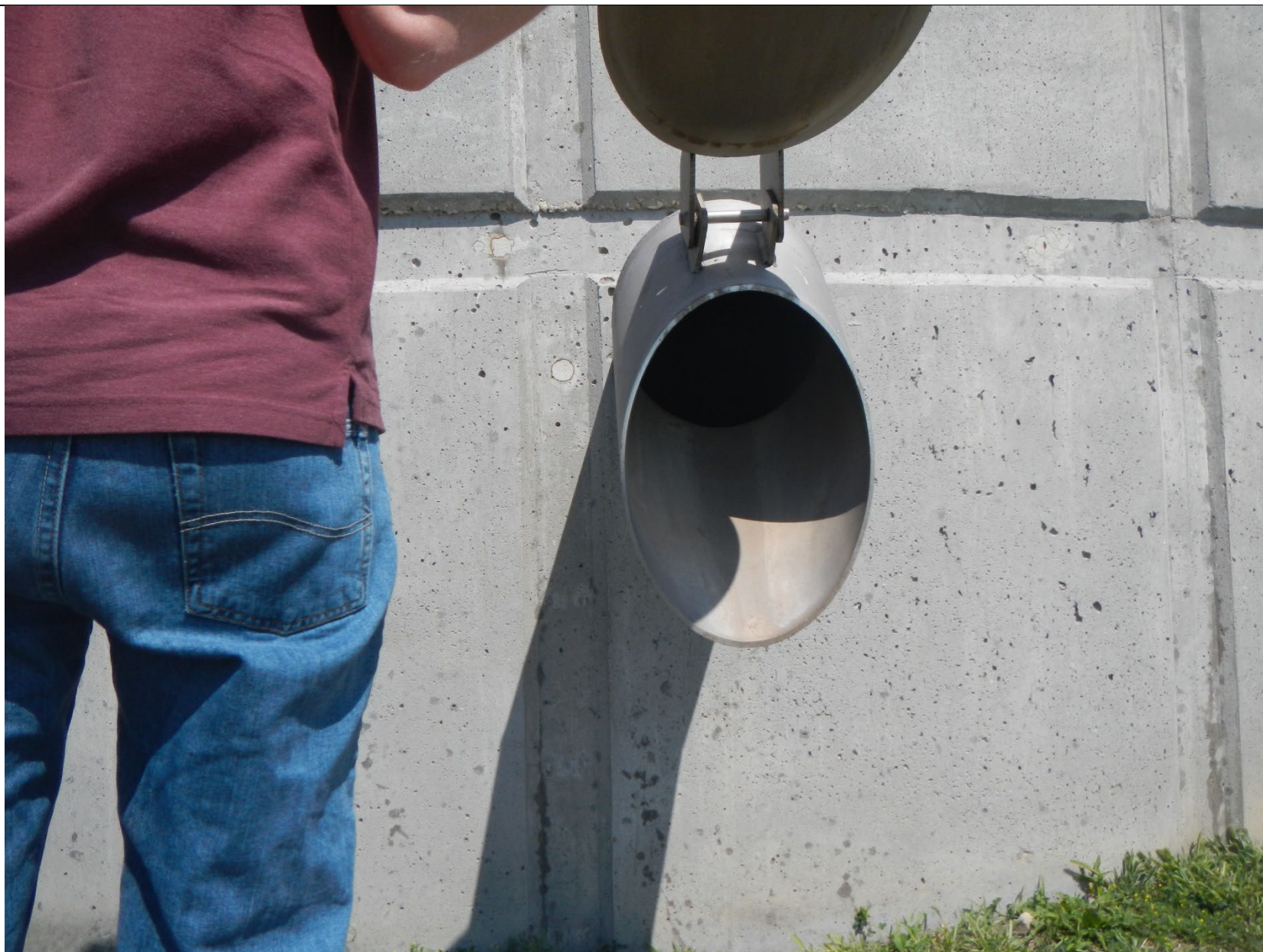
Overflow pipe for Ash Street tower. The overflow had a flapper on it but did not have a screen.
