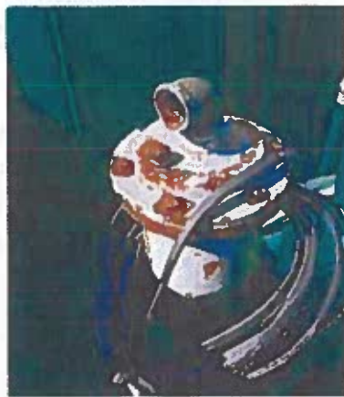
Well #15, air release valve not screened
