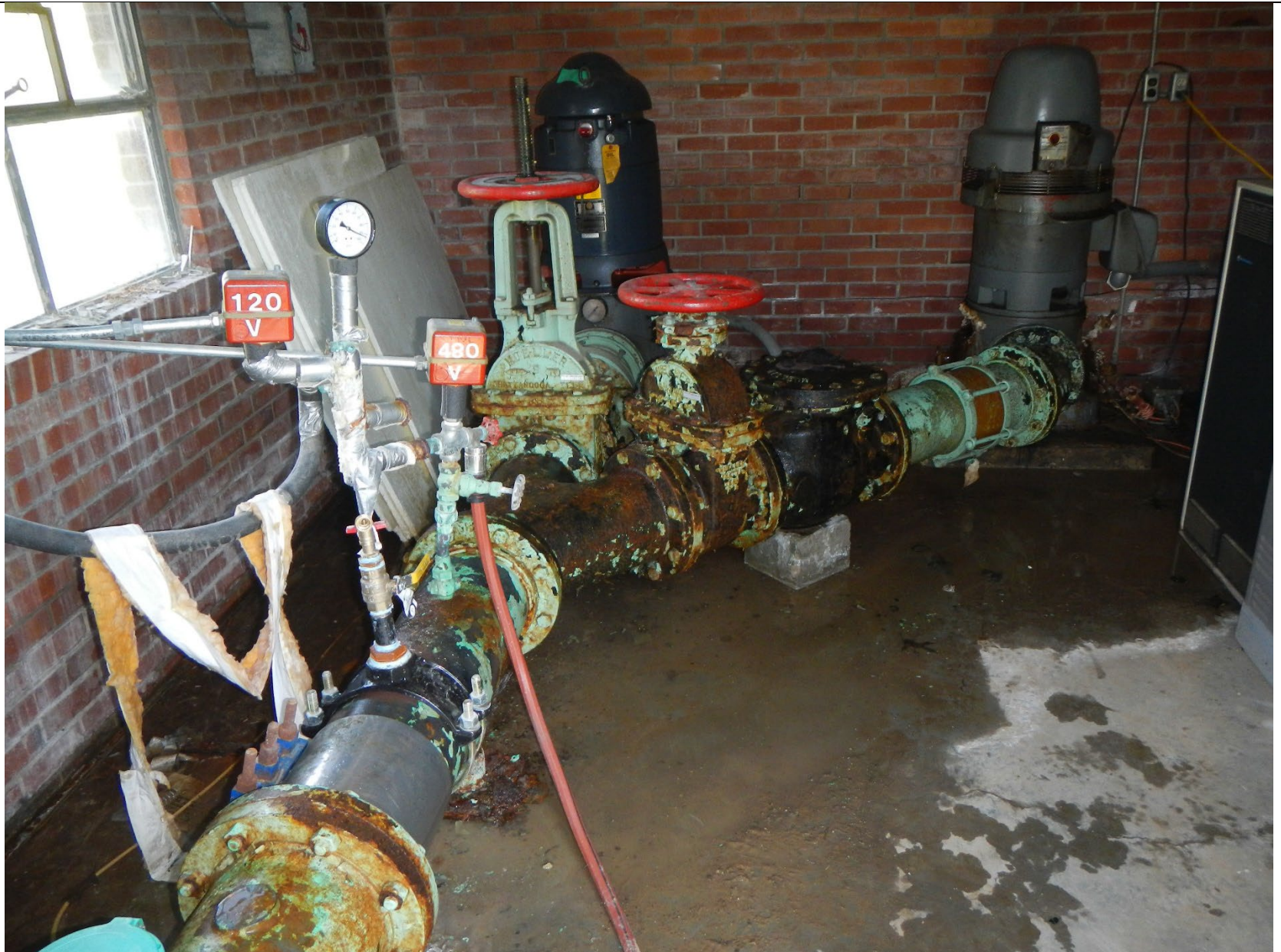
System's booster station. The pump on the right is the one with the leaking packing. The water on the floor is from the leaking packing and was running out the door.
