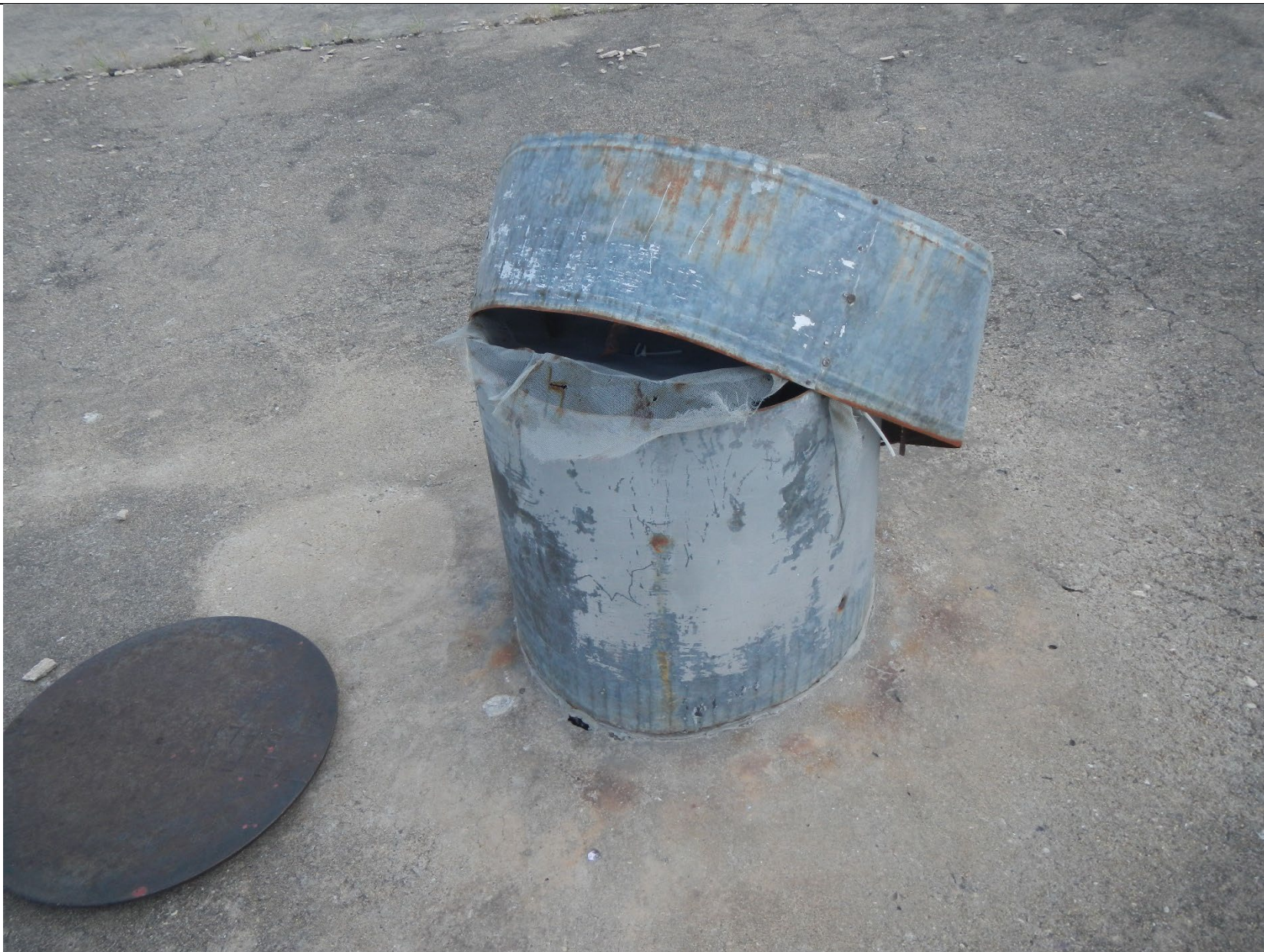
South ground storage tank vent. Vent cover is partially knocked off. Screen is coming off around the front of the vent.
