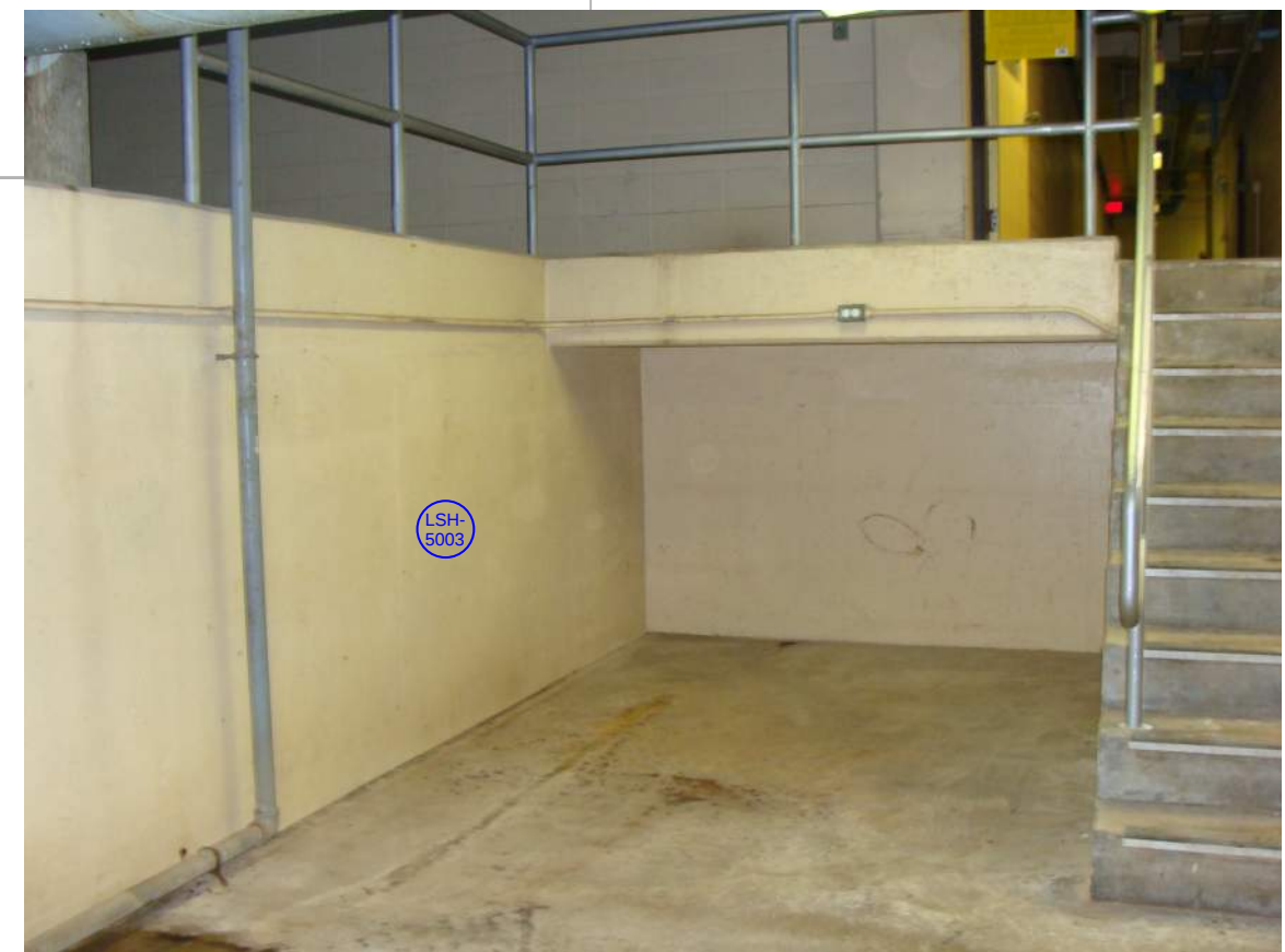
PHOTO 1: LSH-5003 MOUNTING LOCATION
